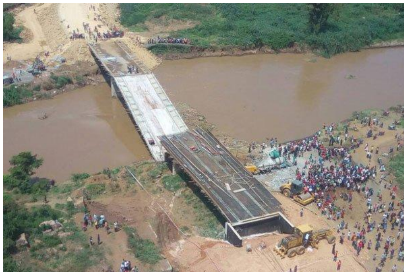
Sigiri Bridge in Budalang'i Constituency collapsed on 26 June 2017
