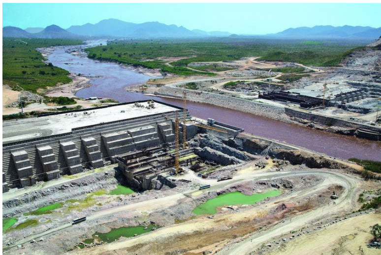
The Grand Ethiopian Renaissance Dam, under construction on the Blue Nile, will be the largest hydroelectric power plant in Africa
